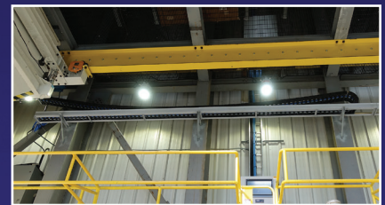
A cable management system protects all wiring and hoses. Electrical power cables are separated from signal cables to protect signal integrity.
